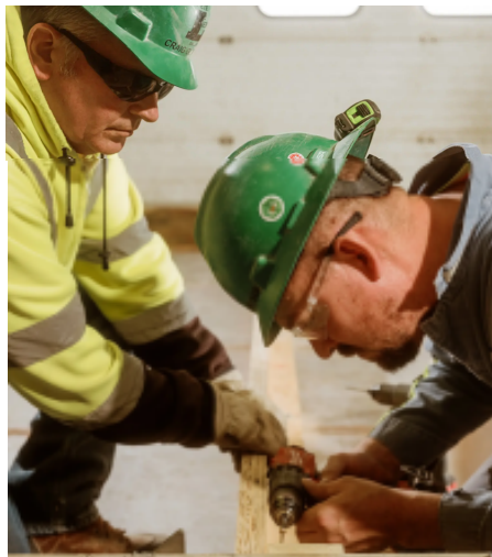
Pete Lien & Sons employees prepared a concrete form that would be poured and assembled into a wall. A green hard hat sticker shows that its wearer prefers quality time. Matthew Defeo for The New York Times
